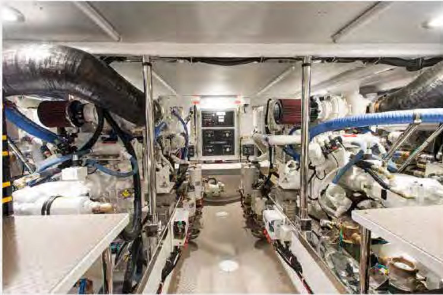
We dedicate more space than most to the engine room simply because it is, of course, the most important part of the yacht.
