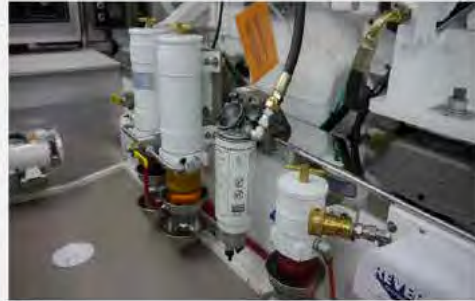
Readily accessible fuel filters
