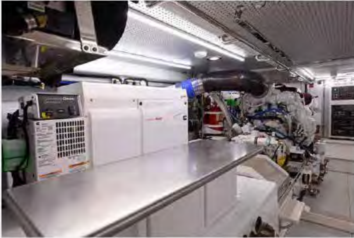
A workbench and air conditioning make the engine room a practical and comfortable workshop
