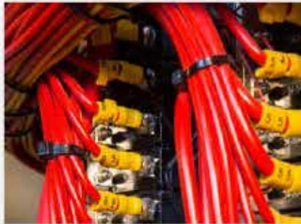
Oversized tinned copper cables
