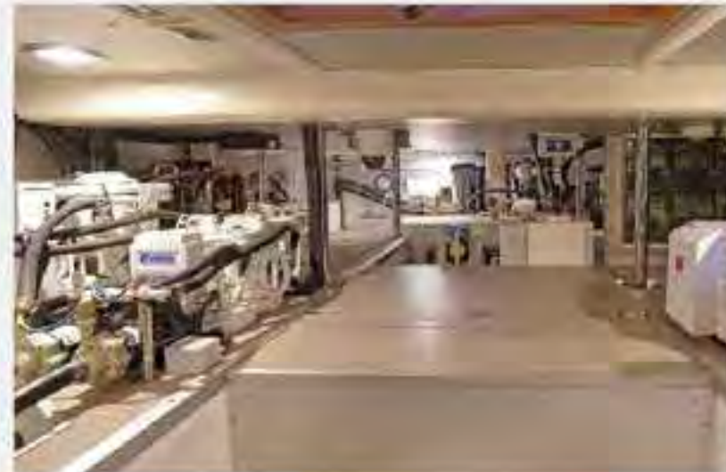
Machinery space under accommodation.
