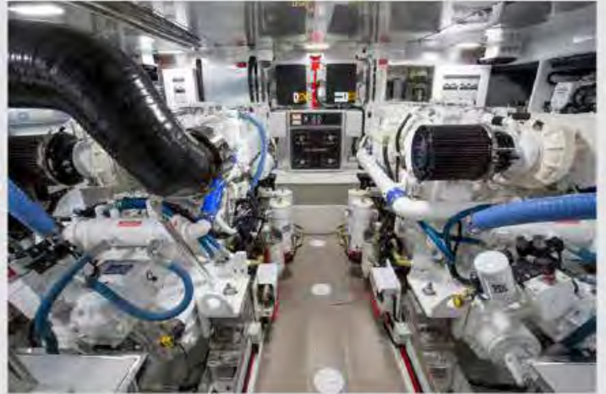
Fleming 58 Engine Room - Twin MAN 800 engines
